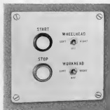
Figure 17B Electrical Controls Right Side of Base
